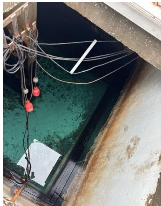
Figure 5-10. Chlorine Contact Basin
