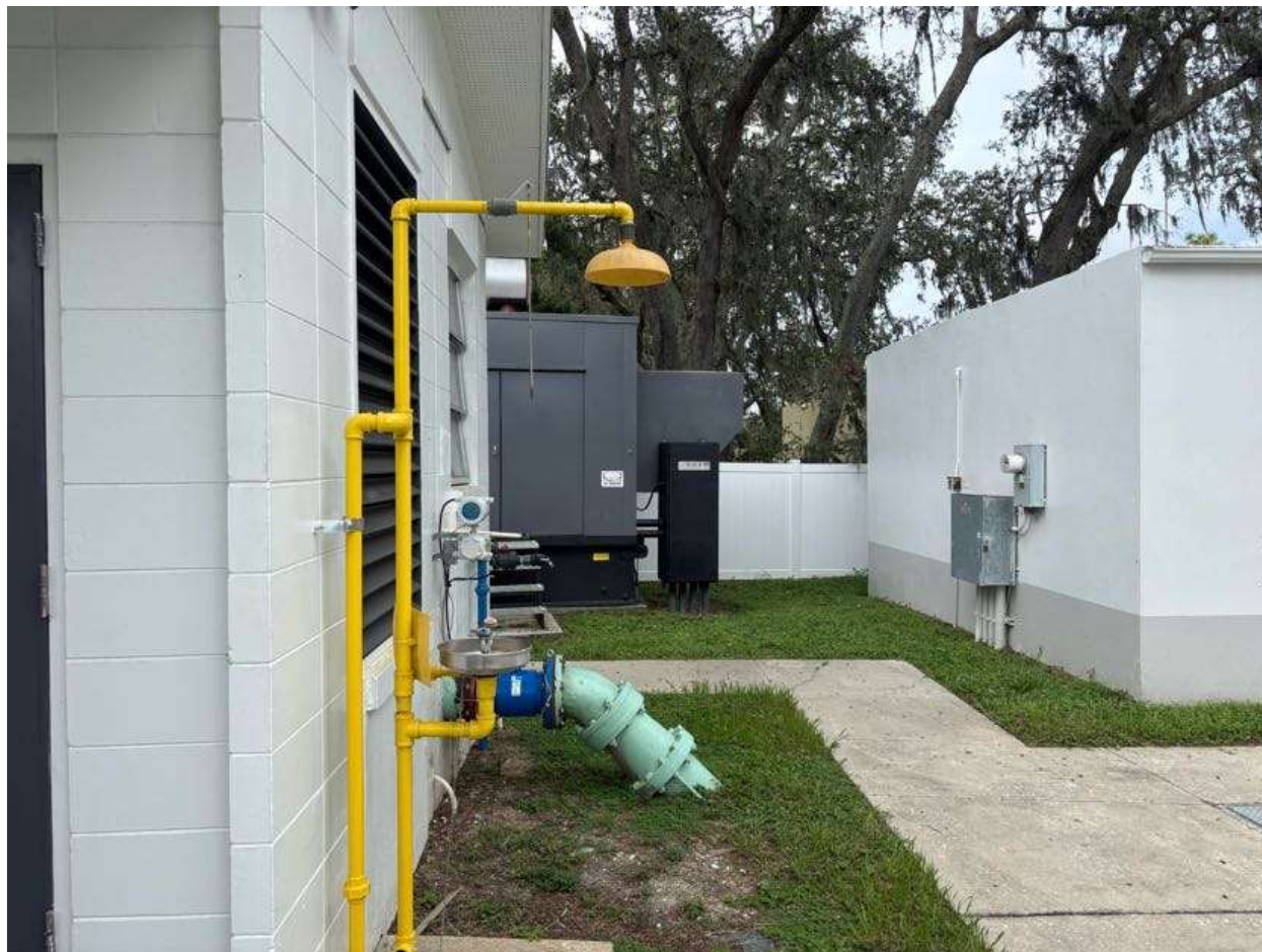
Figure 2-17. Sunningdale WTP Safety Shower/ Eyewash
