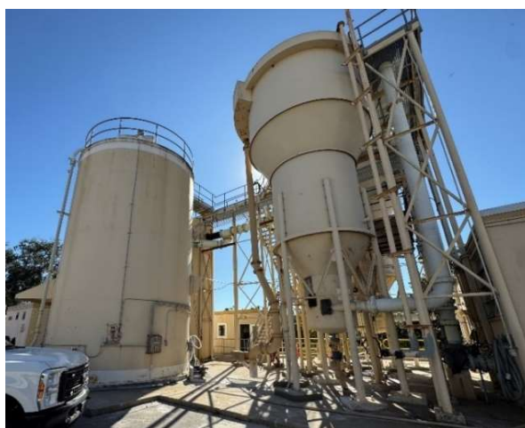
Figure 2-12. Exterior of Gyratur Reactor (Right) and Recarb Tank (Left)
