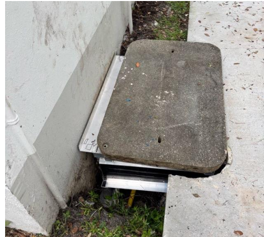
Figure 5-9. Flow meter box
