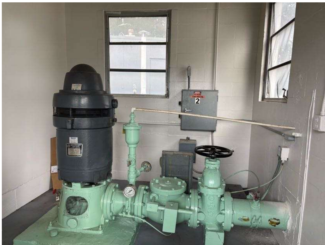
Figure 2-23. Production Well No. 2
