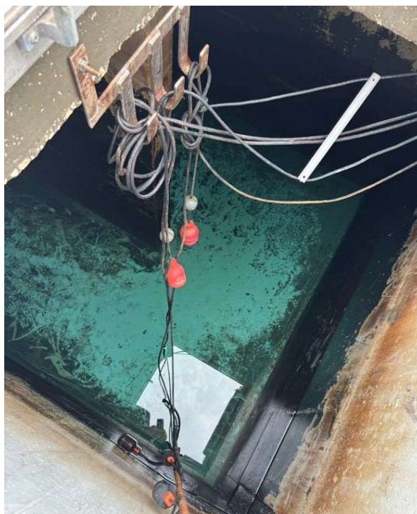
Figure 2-21. Chlorine Contact Basin
