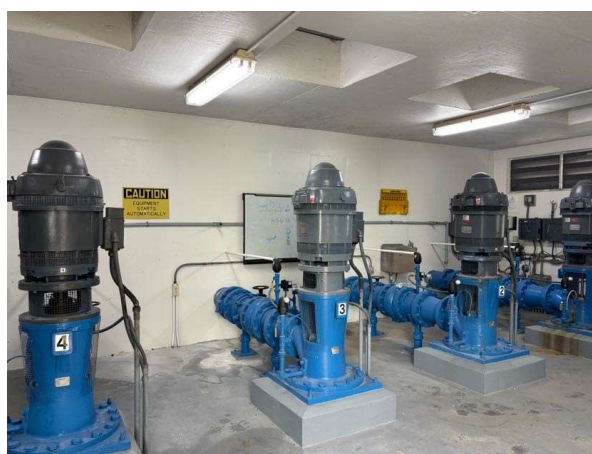
Figure 2-22. Sunningdale High Service Pump Room
