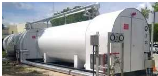
Figure 2-13. Recarbonation System from City of Boca Raton
