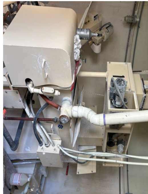
Figure 5-2. Lime Slaker & Slurry System
