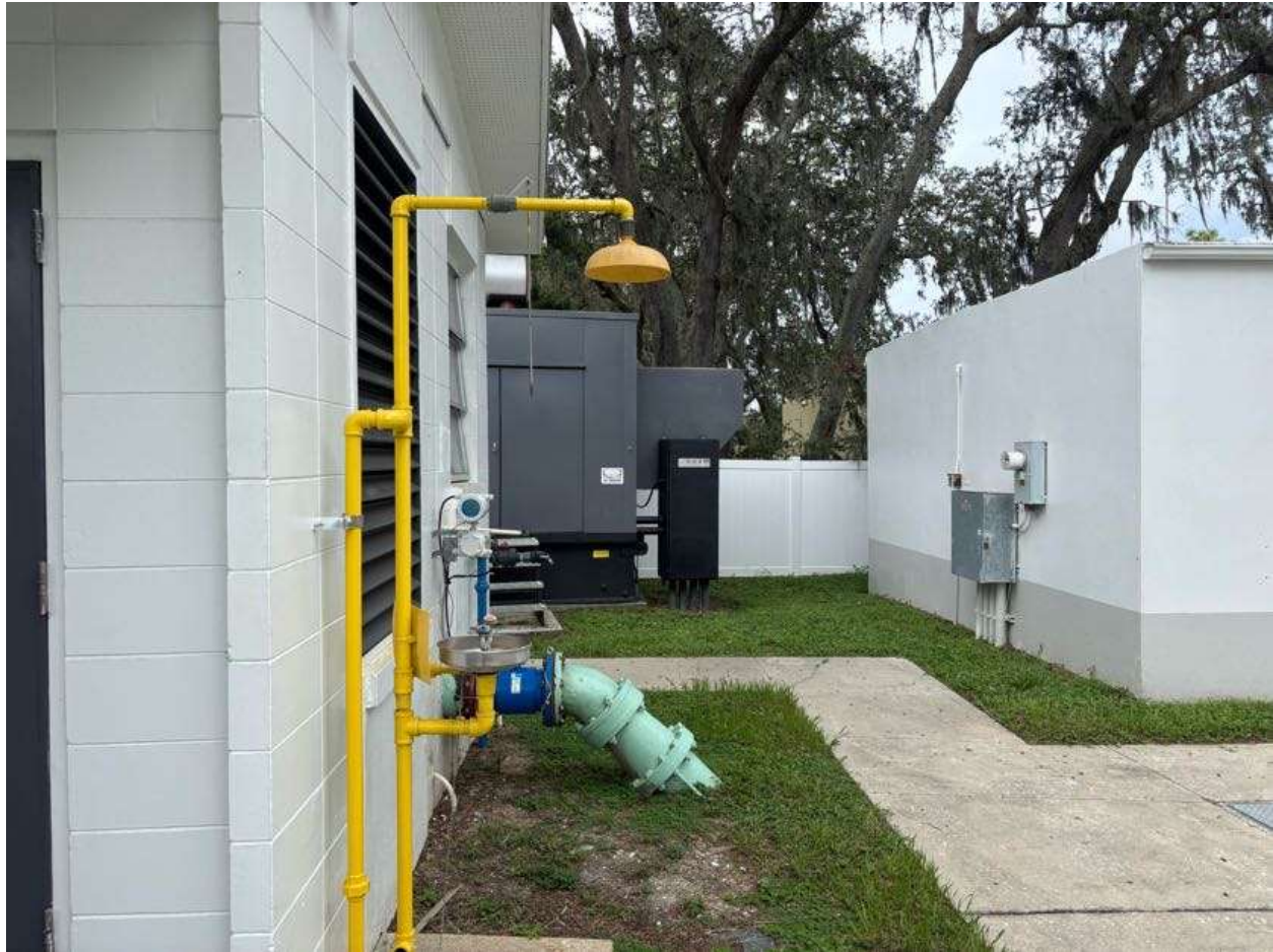
Figure 2-17. Sunningdale WTP Safety Shower/ Eyewash
