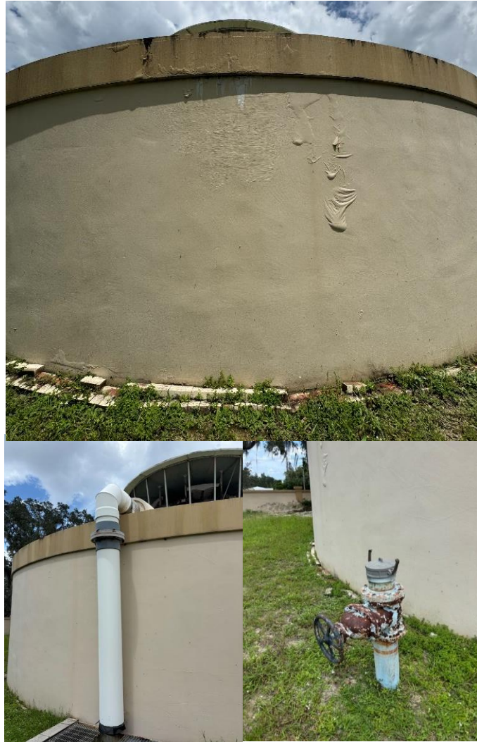
Figure 5-1. Aeration Tank Deficiencies
