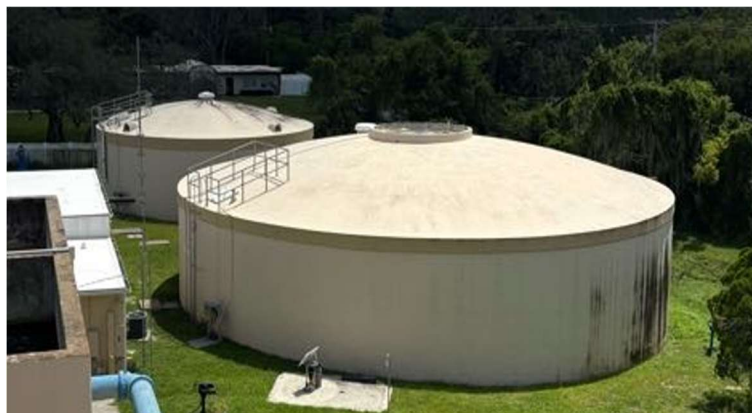
Figure 2-16. 0.2 MG (Rear) and 0.5 MG (Front) “Back Tanks”
